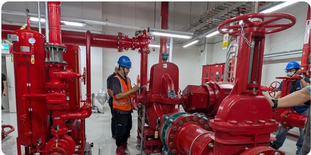
Conducted regular testing of fire protection systems to ensure proper operation
