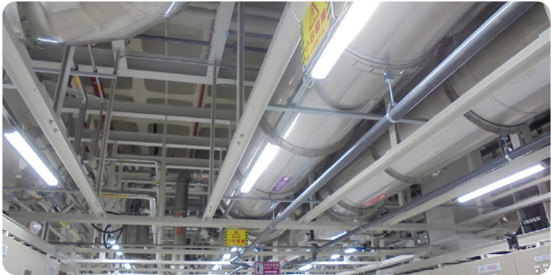
Installed stainless steel ductwork to reduce fire load and prevent fire spread
