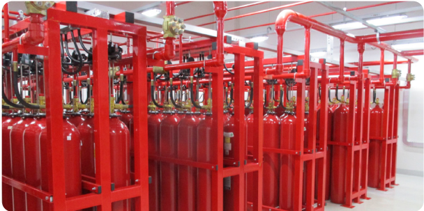
Installed automatic gaseous fire suppression systems
